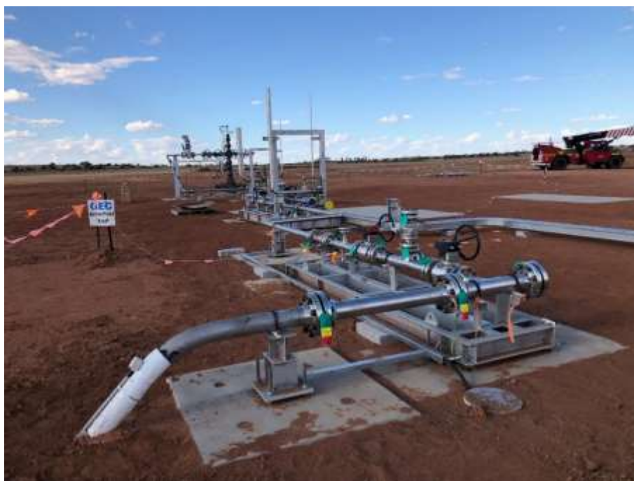
Vali-1 lease skids, with outlet skid in the foreground
