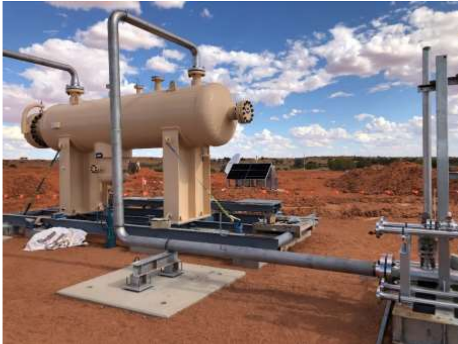
Separator installed at the Vali metering lease
